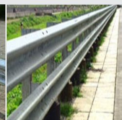
Single Sided Double Beam Crash Barrier
